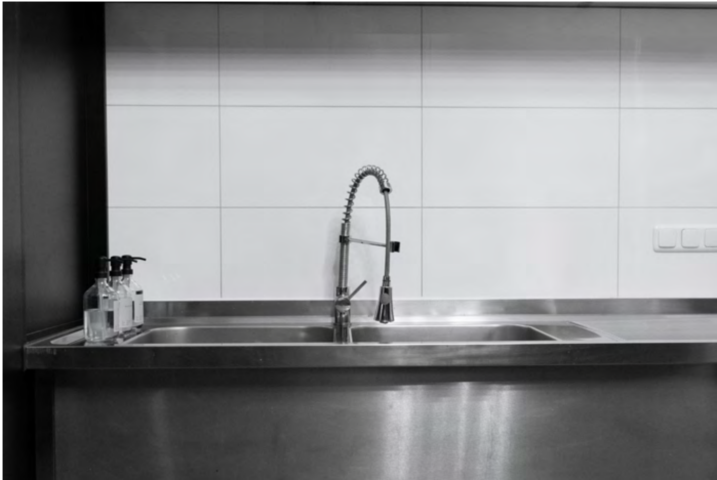
The workshop room additionally serves as a catering room, as it is equipped with a stainless-steel wash and rinsing sink.
